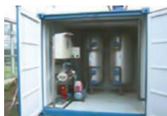
Containerized Equipment Room
