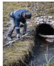
Sewer Cleaning System
